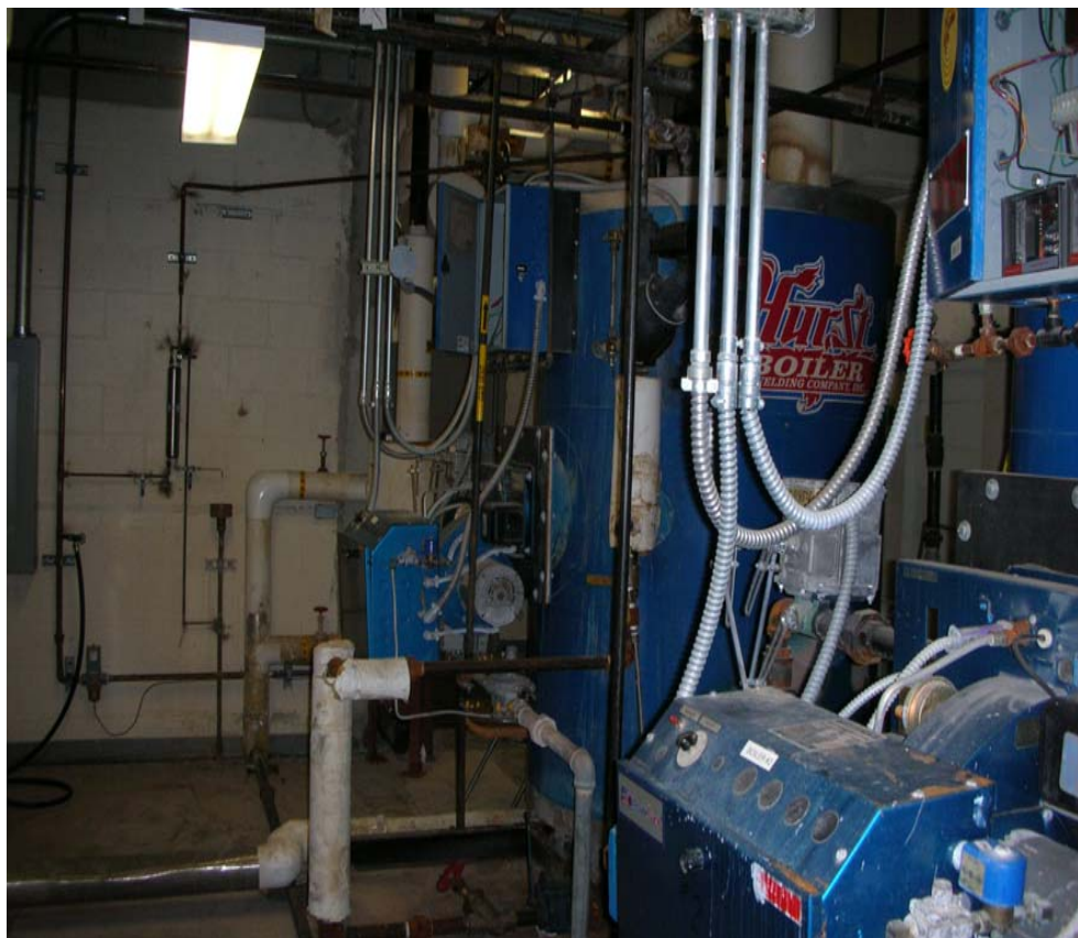
Picture of existing boilers
