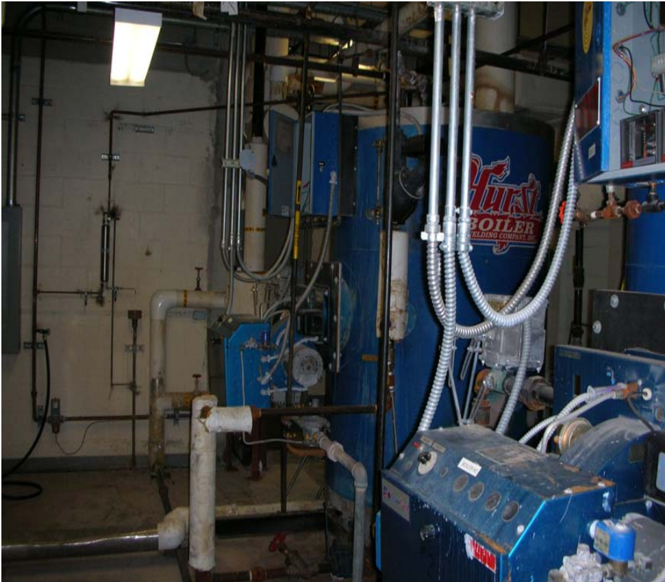
Picture of existing boilers
